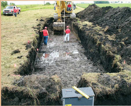
Figure 4. Excavation for a bioreactor installation (courtesy of the Iowa Soybean Association Environmental Programs and Services)
