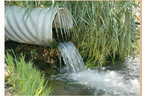
Figure 1. Subsurface tile drain outlet (courtesy of the Leopold Center for Sustainable Agriculture, Jerry DeWitt)
