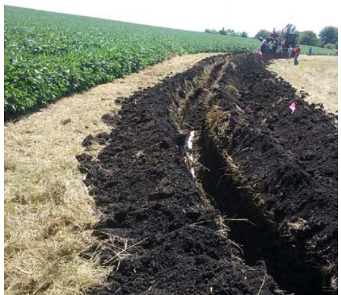
Figure 5: Installation of a saturated buffer using a wheel trencher to lay the distribution pipe.
